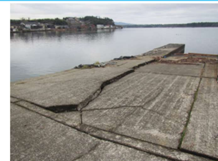
Berth damaged by the earthquake (Ryotsu Fishing Port, Niigata Prefecture)
