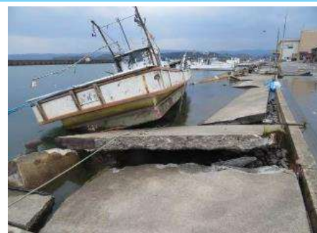
Subsidence and cracking of loading area by the earthquake (Ishizaki Fishing Port, Ishikawa Prefecture)
