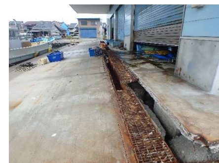
Goods handling facility damaged by the earthquake (Mizuhashi Fishing Port, Toyama Prefecture)
